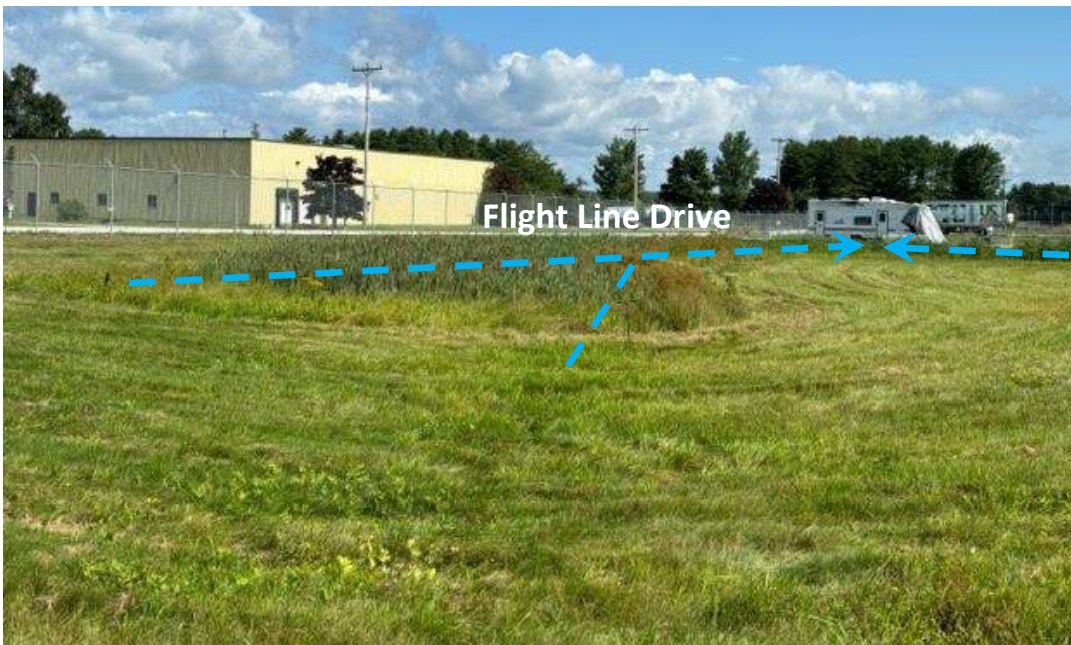
Photograph 4: Northeast overview of the area along Flight Line Drive where surrounding slopes have been graded toward the 18" culvert to capture drainage from the south.
