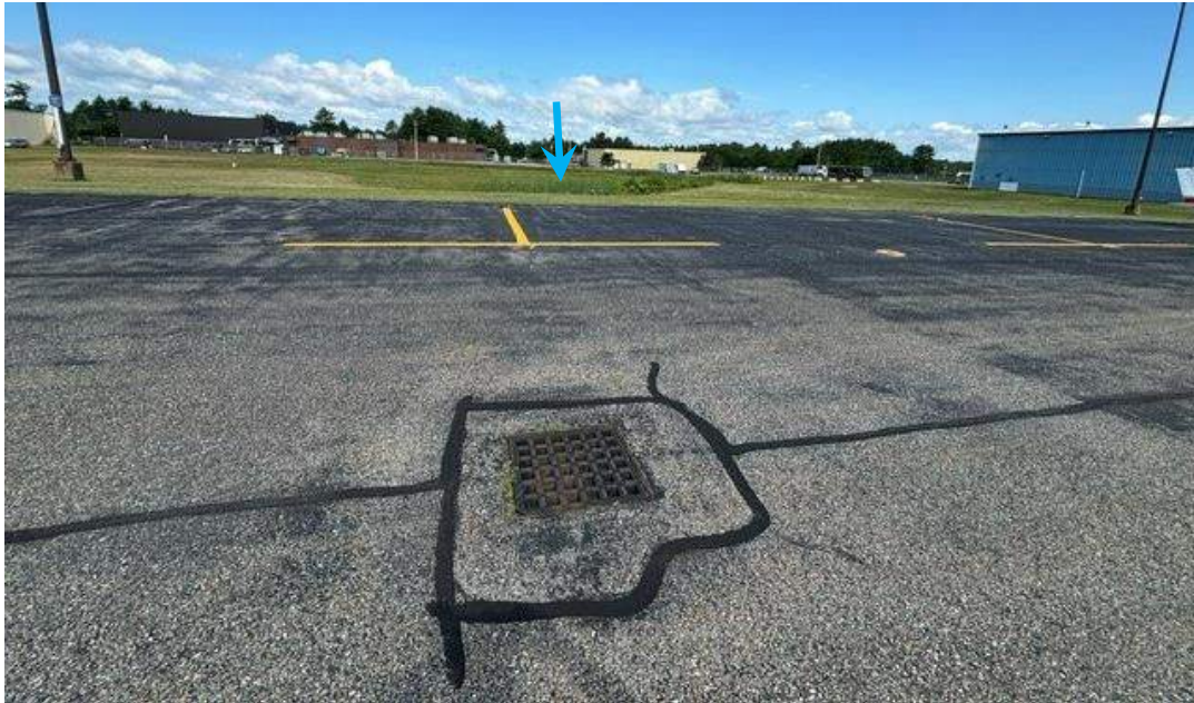
Photograph 1: Westward from aircraft tie down area where the tarmac is drained by a network of catch basins that outfall into a ditch leading to culvert (arrow) crossing under Flight Line Drive.
